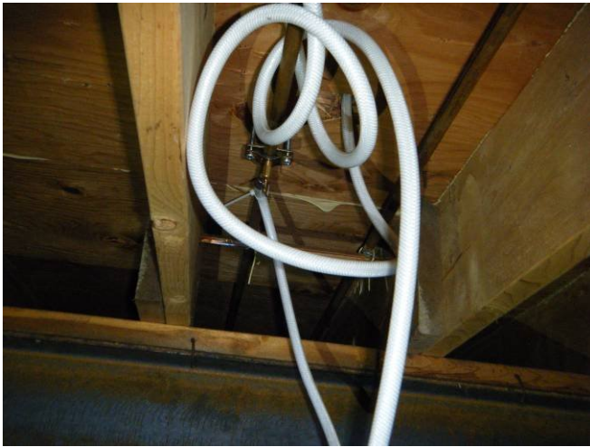
55 Fridge water line
