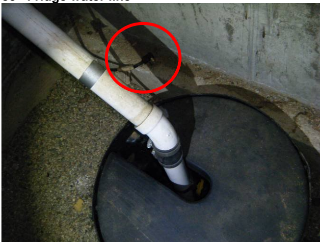
56 Sump not plugged in
