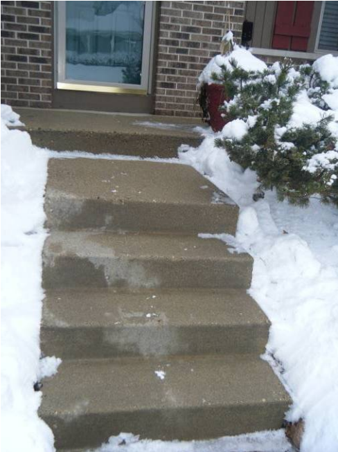
2 Should have a railing
