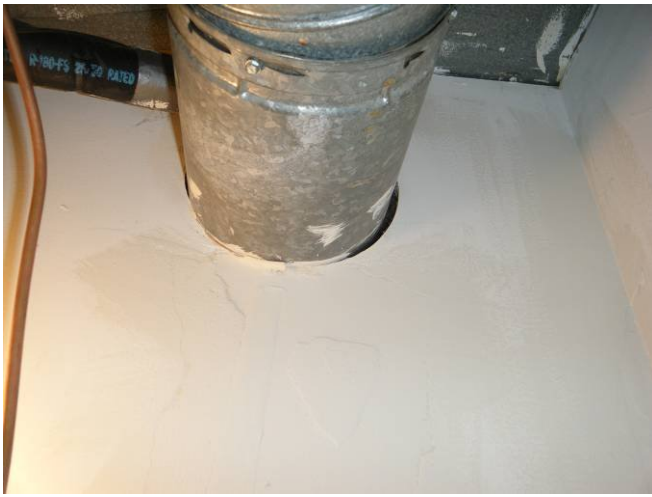
24 Flue in direct contact with drywall. Must have 1-2" of clearance
