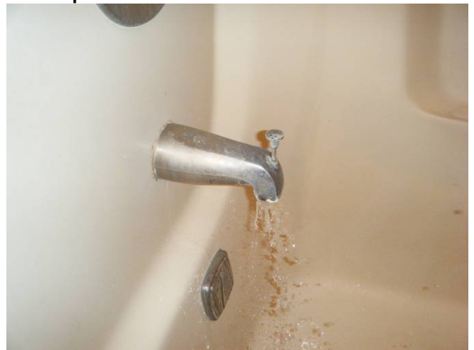
34 Master tub spigot corroded pull. Replace spigot
