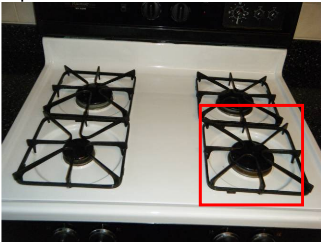
30 Igniter doesn't work
