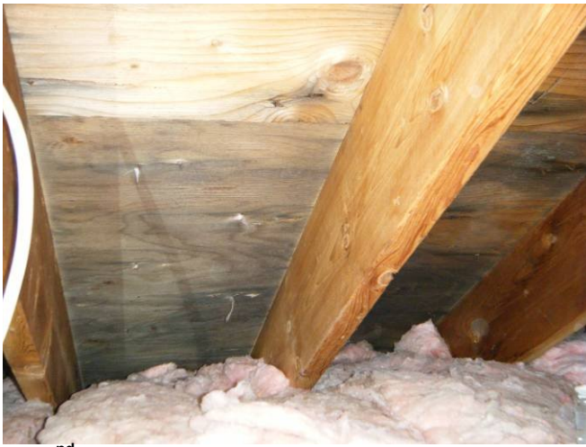
42 2 nd story attic space - mold
