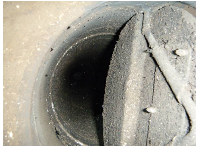
33 Fireplace flue - Time to be cleaned
