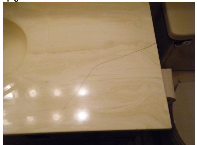
35 Crack in master vanity top
