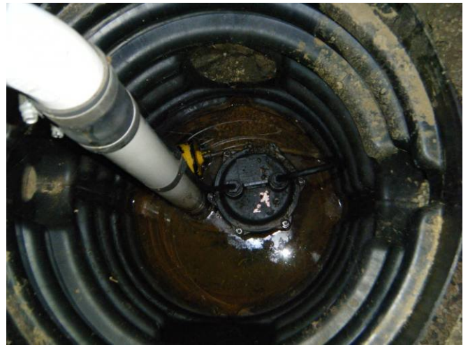
57 Sump pump doesn't work when plugged in
