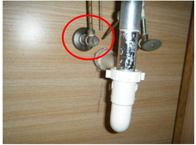
22 Hot water valve stem broken for hot water in powder room
