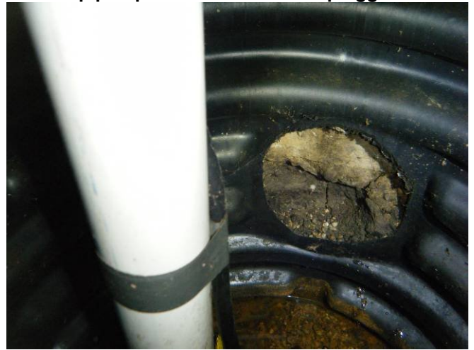
58 No drain tile system
