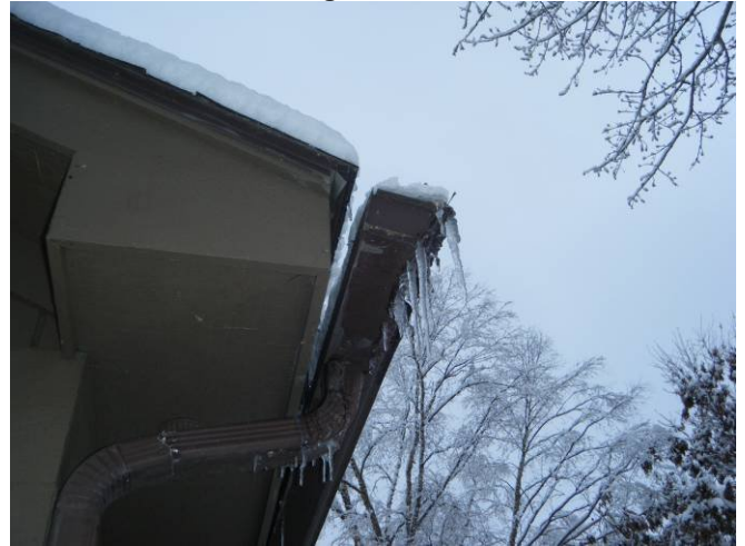
5 Loose gutter in NW corner
