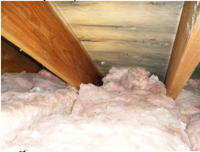
43 2 nd story attic space - mold
