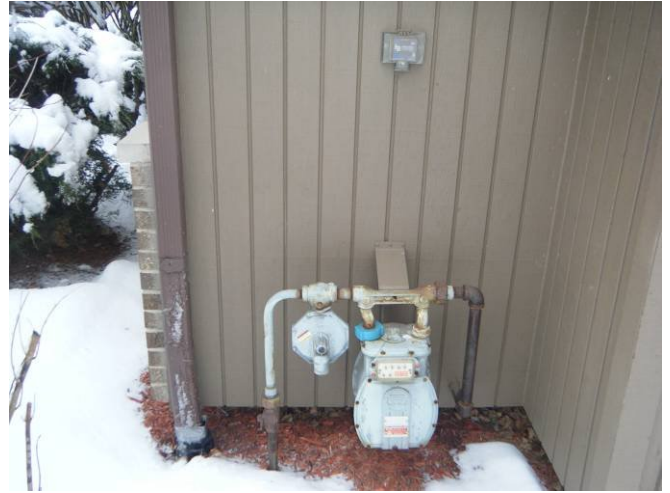
4 Gas meter & sending unit for water meter
