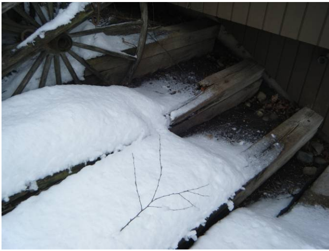
13 Three step retaining wall rotted and leaning
