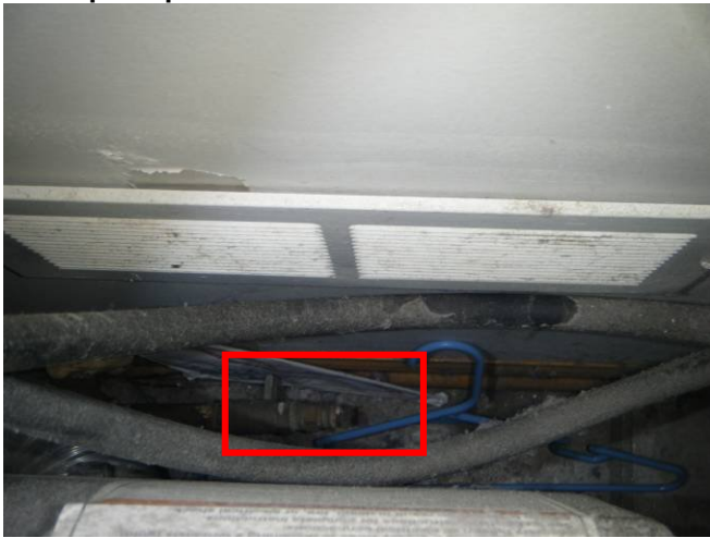
20 Cap unused gas line behind dryer
