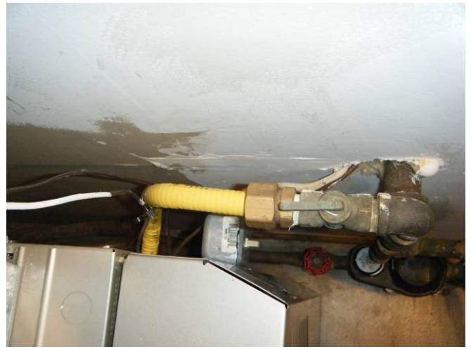
26 Flex gas line on furnace
